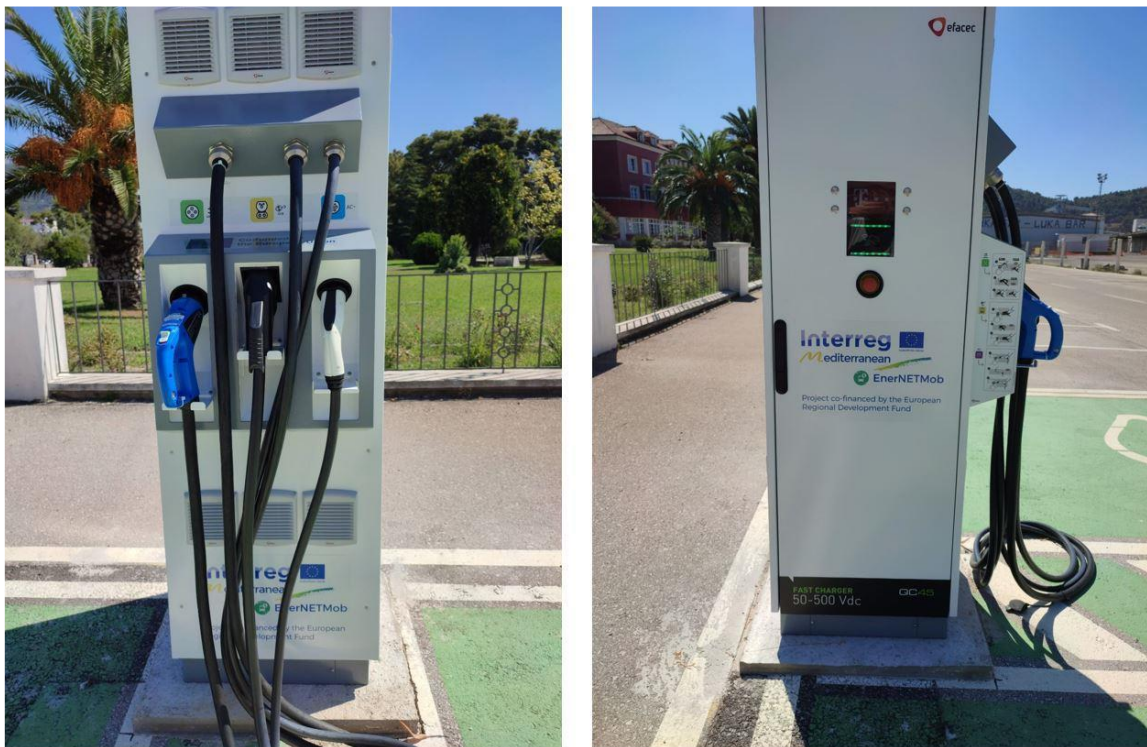
Figure 9: Fast charger installed in front of headquarter of the Port of Bar
